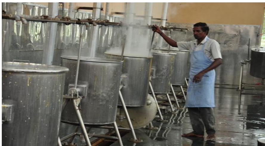
Figure 41 Boilers in centralised kitchen in Lawspet, Puducherry
