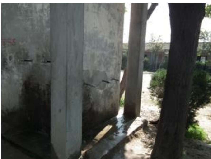
POOR DRINKING WATER CONDITIONS IN A SCHOOL
